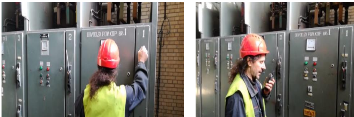
Figure 7. Turning on the power and noting that the system is under voltage
